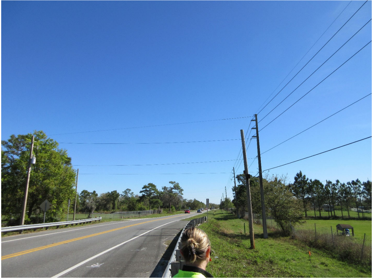
Wood Utility Pole and Concrete Strain Pole
