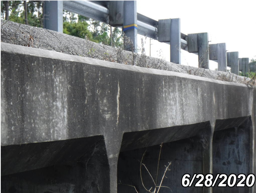
Photo 3: Element 8475: Vertical crack with efflorescence in north headwall.
