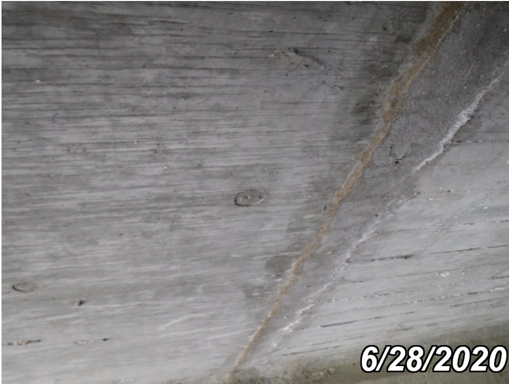
Photo 5: Element 241: Patched crack with efflorescence and rust staining in the underside of Cell 2 at the cold joint.
