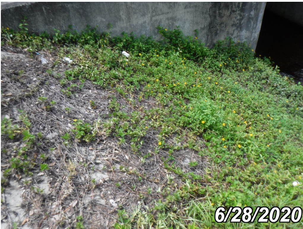
Photo 6: Element 8394: Heavy vegetation growth on the southwest slope protection.
