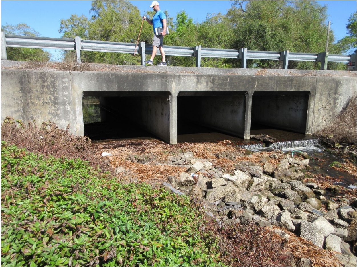
Culvert Downstream showing debris in Barrel
