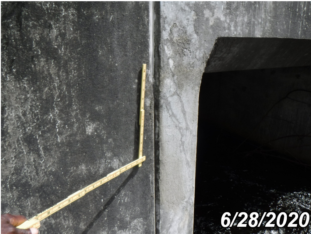
Photo 4: Element 241: Delaminated patch at the north end of Wall 4.
