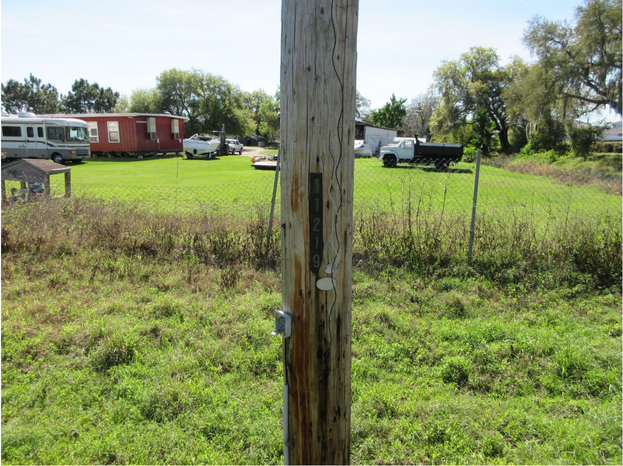
Wood Utility pole
