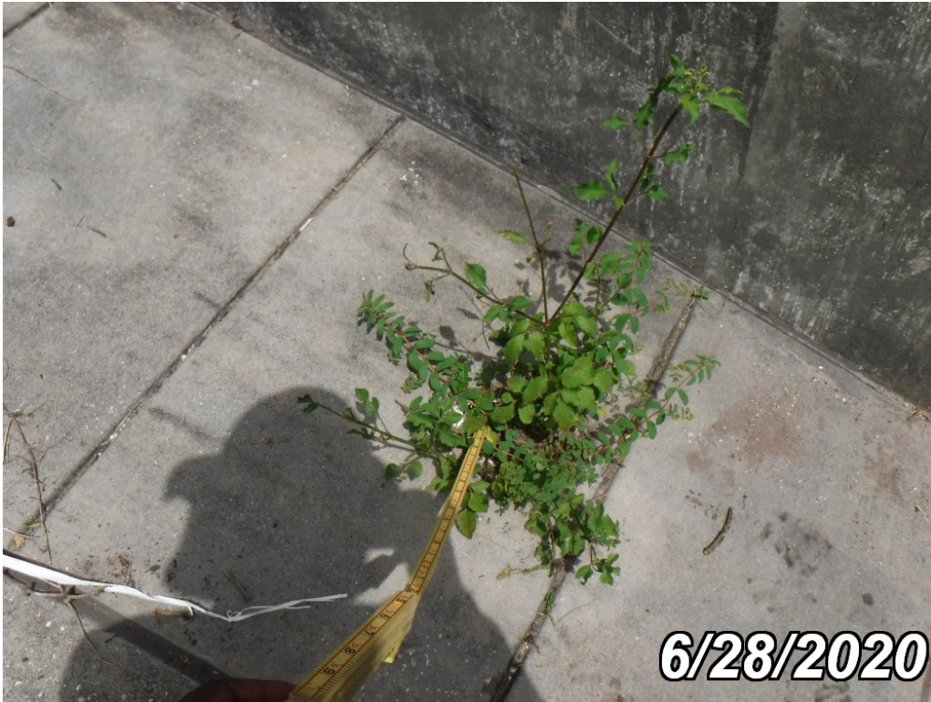
Photo 7: Element 8394: Clogged weep hole at the northwest slope protection.
