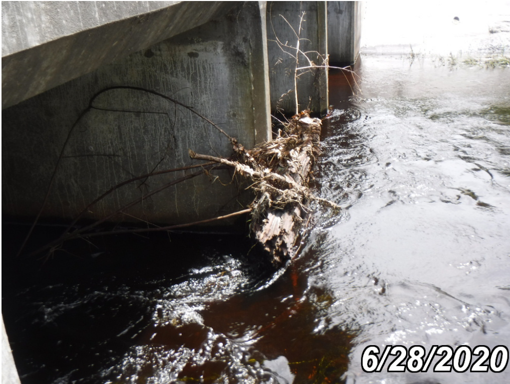
Photo 1: Element 8290: Debris in channel at Wall 3.
